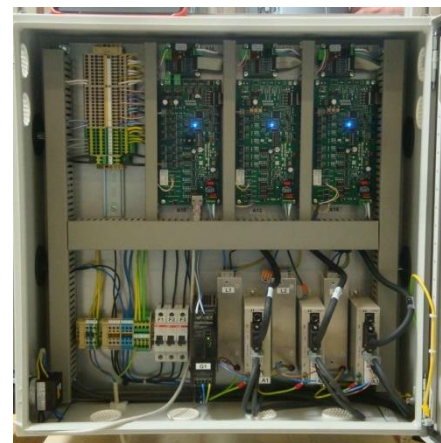
Control cabinet for control of linear coupler
